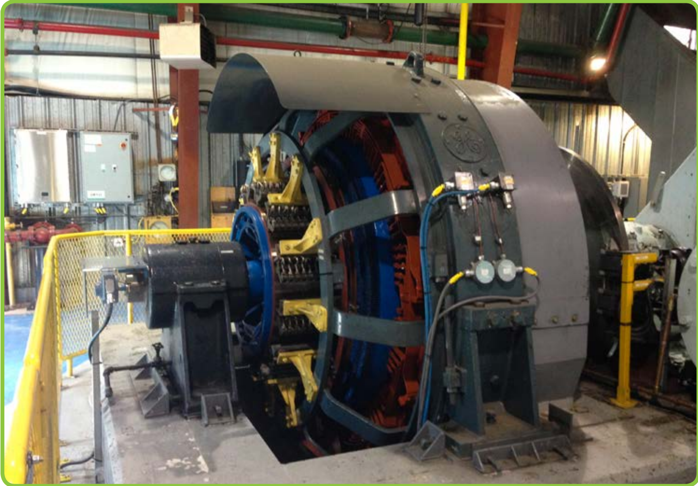
Existing 3,000 hp DC Hoist Motor
